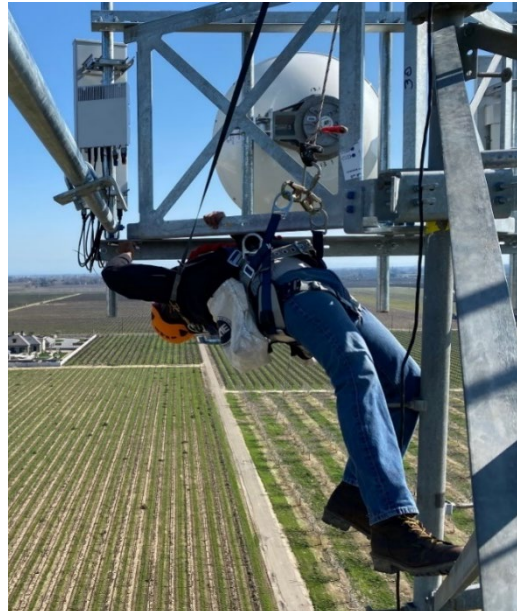
One of our crewmembers deploying new fixed wireless service to an area, showing examples of a sector antenna that serves customers and a microwave antenna that connects to the Internet.
