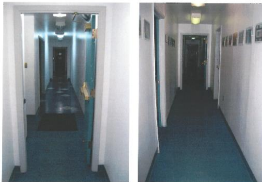
Interior doors without 18" push side clearance
