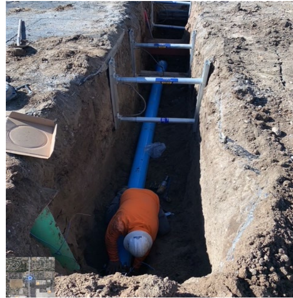
Alpine Drive Water Main
