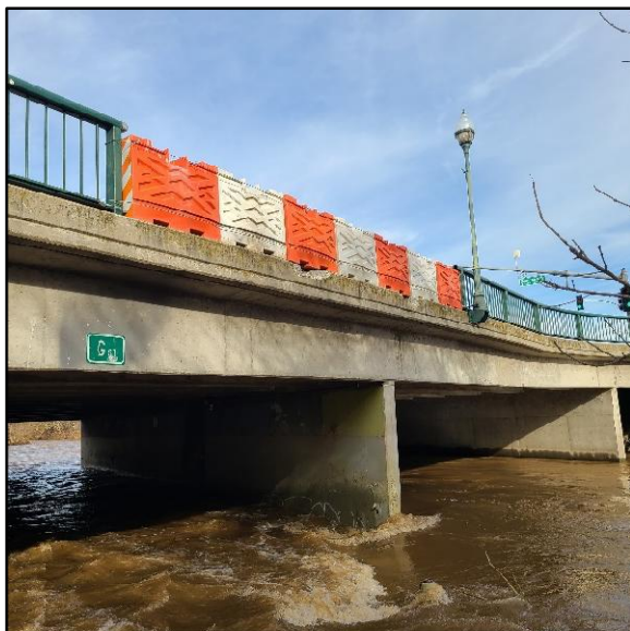
Figure 1: Elevation View of Damaged Railing (Looking West)
