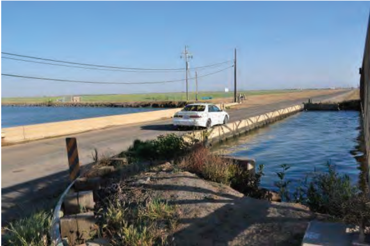
Figure 4-36 Evidence of Gradual Land Subsidence, Partially Submerged Russell Avenue Bridge, Mendota, CA
